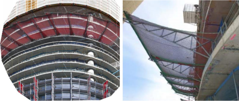
Figure 1-59b: Photographic Example of Perimeter Catch Fan Systems
